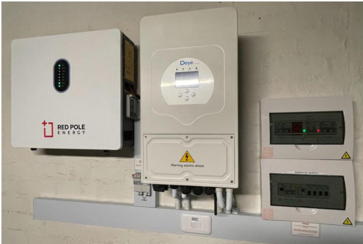
DEYE 5kw installed with 1 x Vital 5 battery
