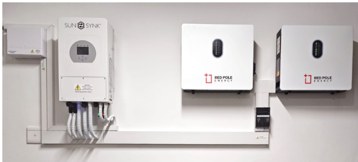
Sunsynk 8kw installed with 2 x Vital 5 batteries
